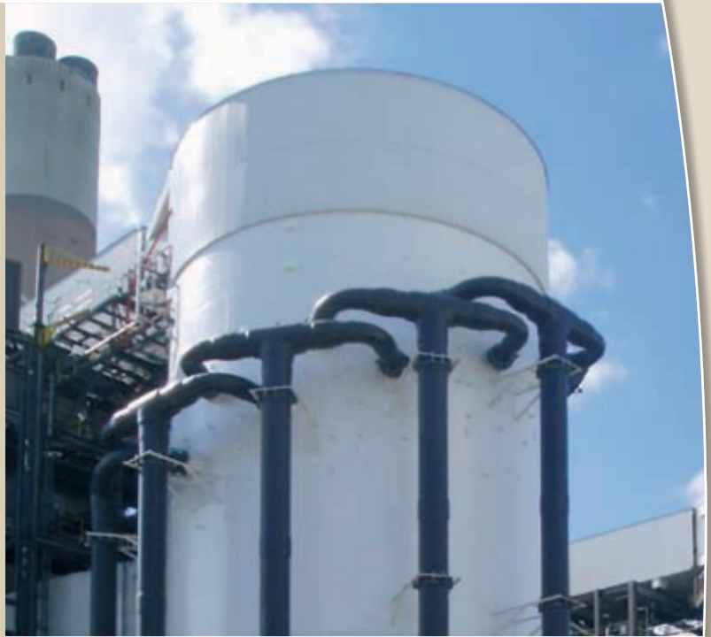
Outer coating of a FGD absorber
