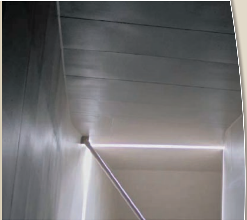
Clean gas duct
